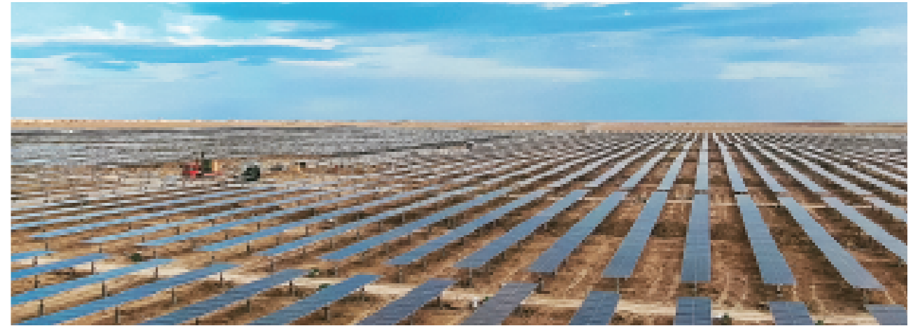
Ground-mounted power station project in Qinghai Province
