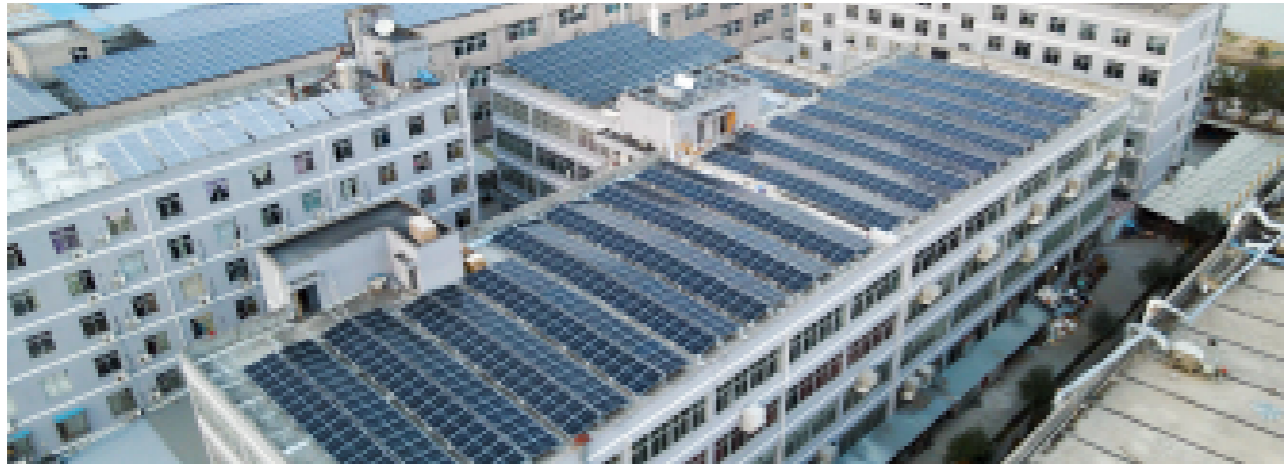
C&I rooftop project in Zhe Jiang Province, China
