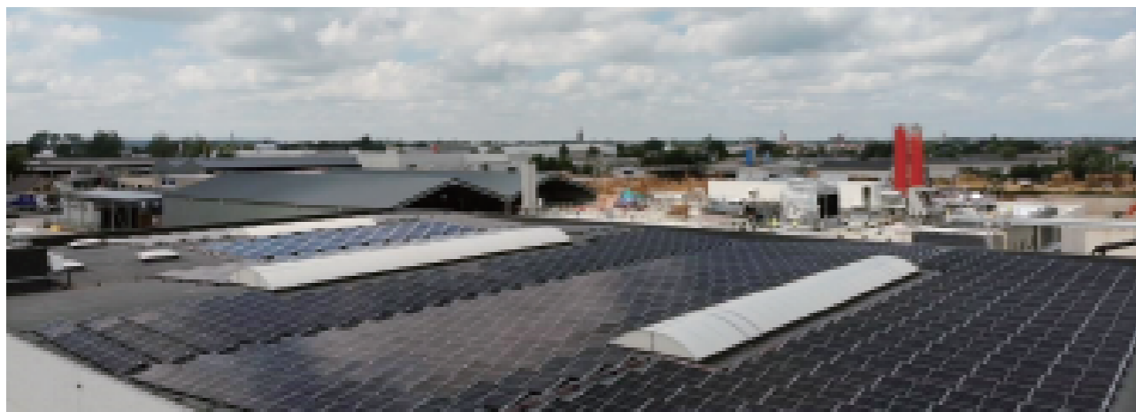
C&I rooftop project in Belgium, Europe
